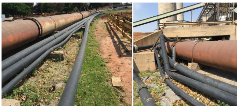
Figure 2-5: Current State of the Pipe Supports on Site
